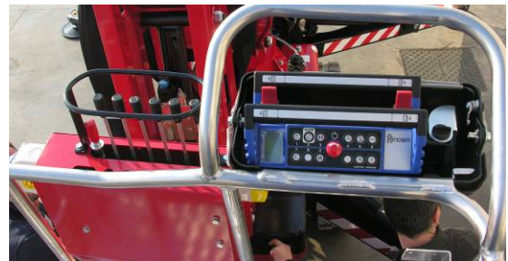
RADIO CONTROL CORRECTLY INSTALLED INTO THE BASKET SUPPORT
