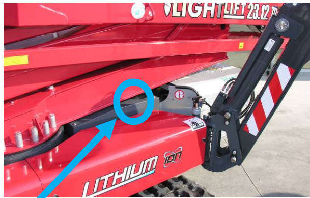
Batteries charger led on 72 Volt batteries pack
