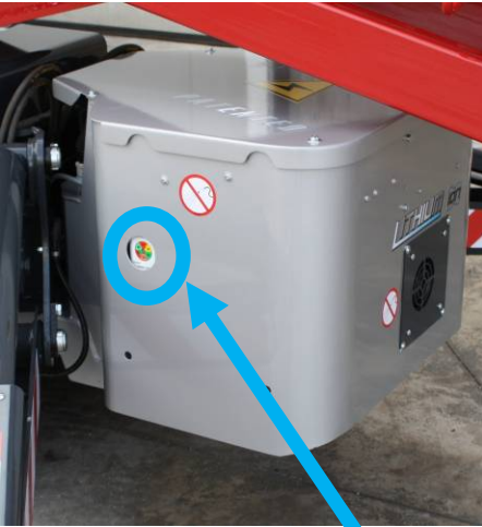
Batteries charger led on 48 Volt batteries pack
